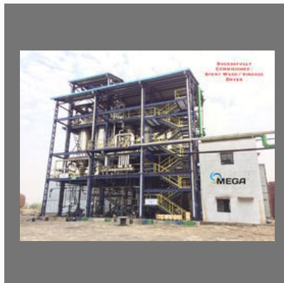
Spent Wash Dryer
