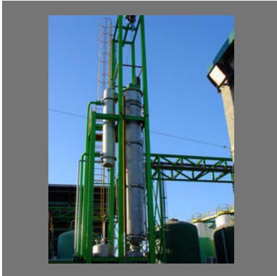
Thin Film Agitated Evaporation Plant
